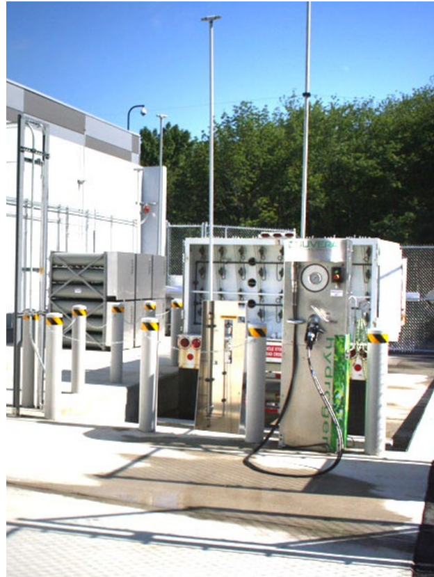
Hydrogen fueling dispensers are the size of a standard gasoline pump and occupy minimal space.
